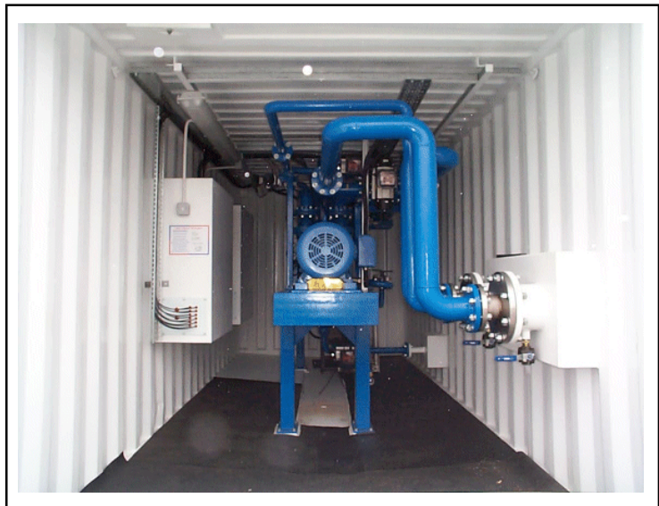
Electric Powered Twin Liquid Ring Vacuum Unit
